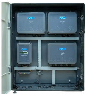
Interior View of xMasm10 - Wired Solution
