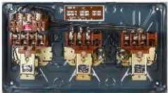
Interior View of MK2 SASD
