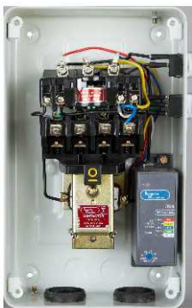
Interior View of MK1.i
