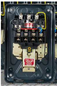
Interior View of MK1 DOL
