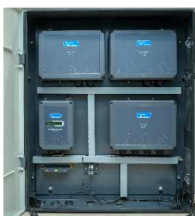
Interior View of xMasm10 - Wired Solution
