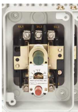
Interior View of MF1 DOL - 3Ø Starter
