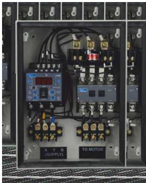
Interior View of MD Starter+ DOL Starter
